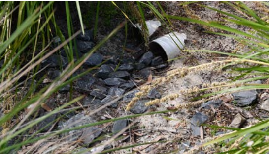
Stormwater management raingarden
