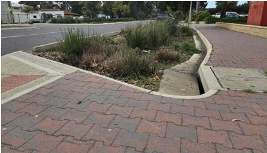
Raingarden side entry pit
